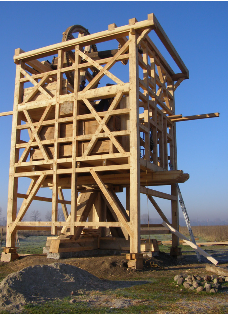
Fig. 18: A windmill from Zawada during reconstruction at the Łęczyca Croft in Kwiatkówek; the timber-frame structure was entirely recreated from new material; photo by F. Tomaszewski, November 2011.
