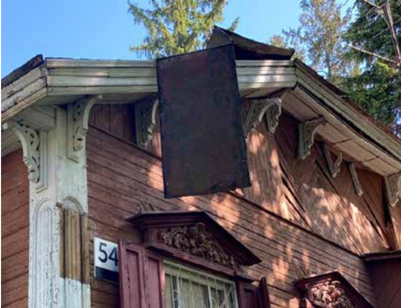
Figure 7: Damage to the corner fragment of the facade of the “wooden Art Nouveau” style mansion. Photo by A. Hlushchenko
