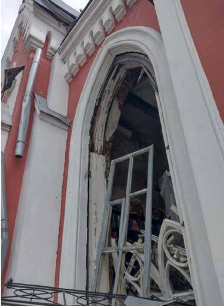
Figure 5: Destroyed window of the courtyard facade. Photo by A. Glushchenko, 2022
