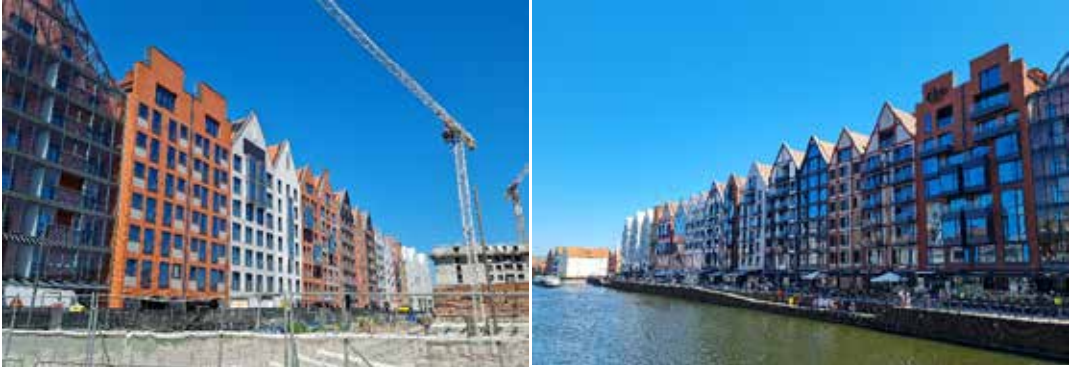
Figure 10 a, b: View of the reconstruction of Granary Island in Gdansk. Photo by D. Kuśnierz-Krupa
