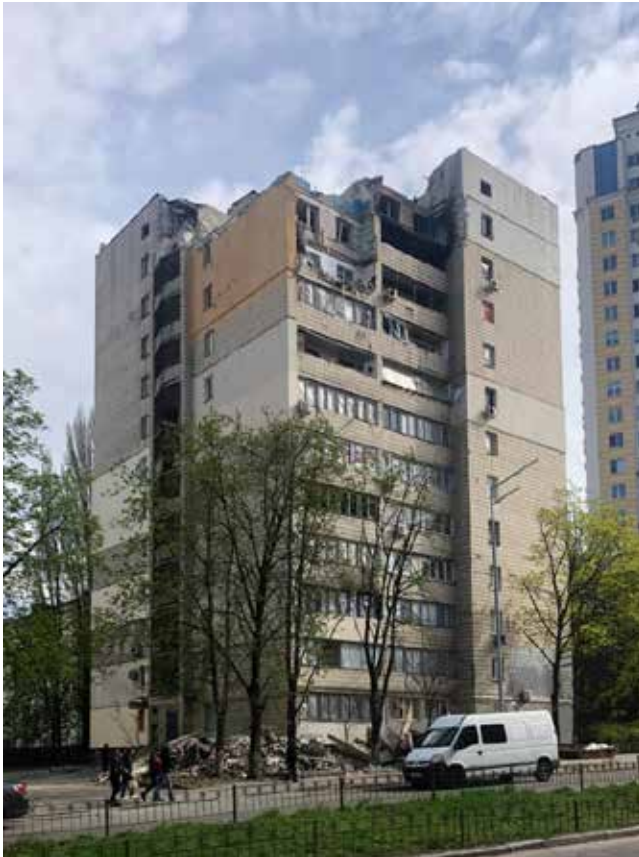
Figure 1: Destroyed upper floor of the residential building in Kyiv. Photo by Yu. Ivashko, 2022
